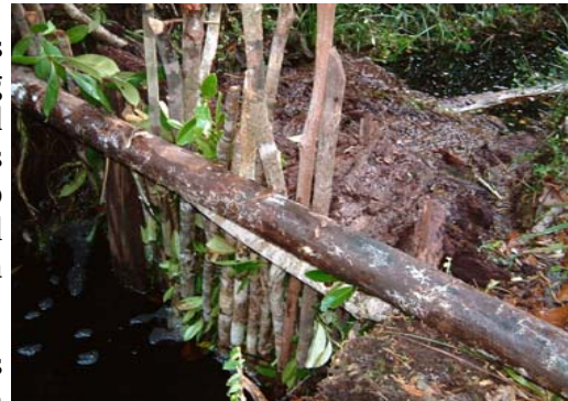
Dam in illegal logging canal in the Sabangau catchment, Central Kalimantan, Indonesia, constructed using local available material although simple the dam is effective as a water management strategy that mitigates carbon loss
